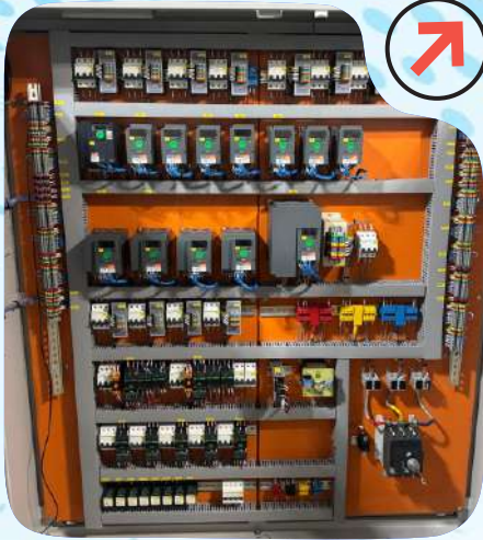
AC Drive panel
